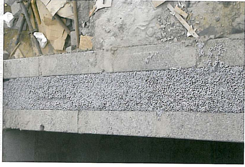
Polypearl infill of 150mm cavity in one of the houses at Castlemagner.
