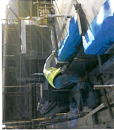
First floor joist made airtight at the Magner Development Ltd scheme in Castlemagner, Co Cork .
